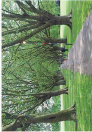
Photo B, above, shows the existing footpath and the extent of damaged ground.
