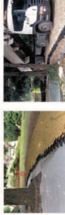
Images above show the type of build up that would reduce impact on existing trees
